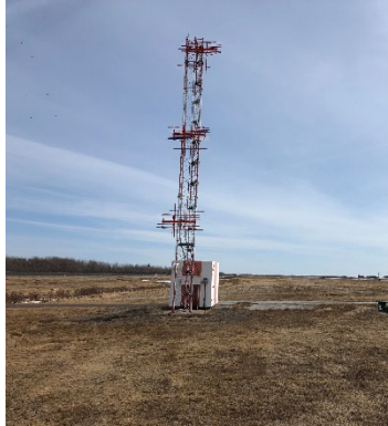
Photo 2: Glide Slope Antenna
