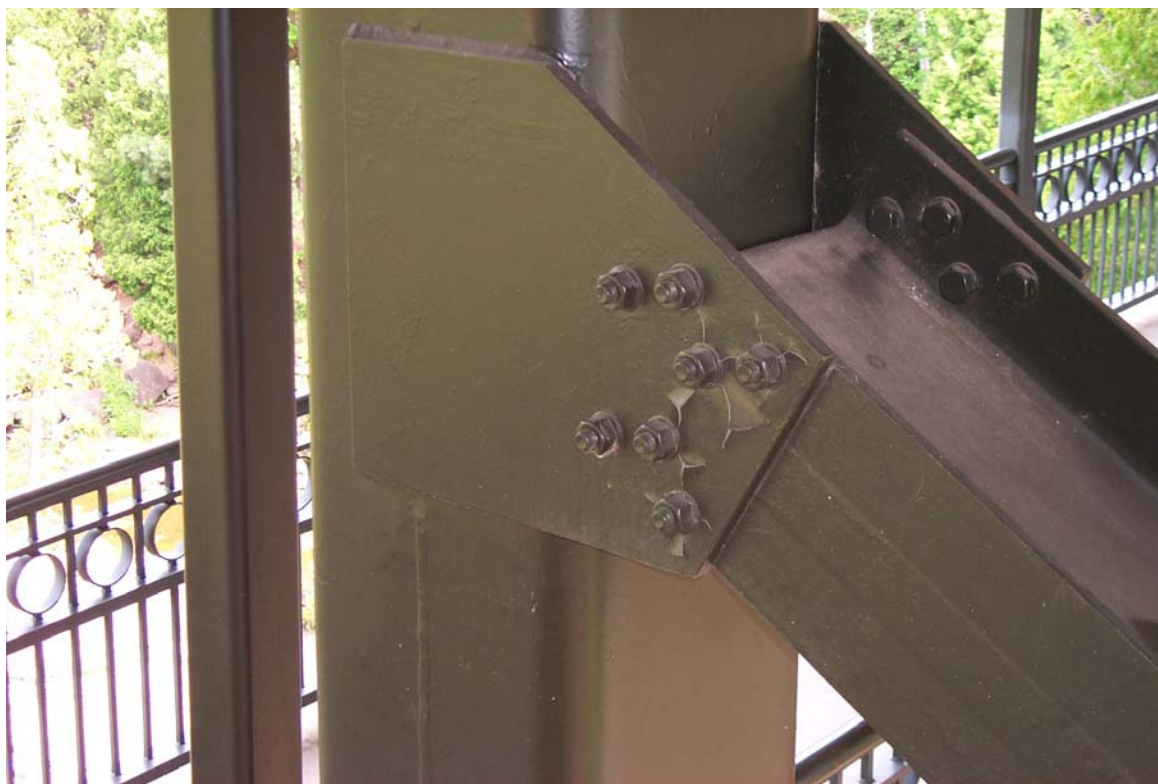
Photo #3: Paint failure on pier bracing connection (typical)
