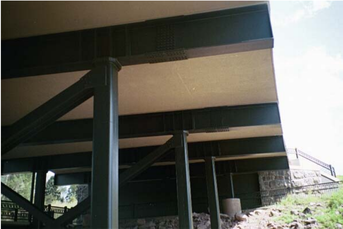
View of north approach spans - note pier cap splices due to staged construction.
