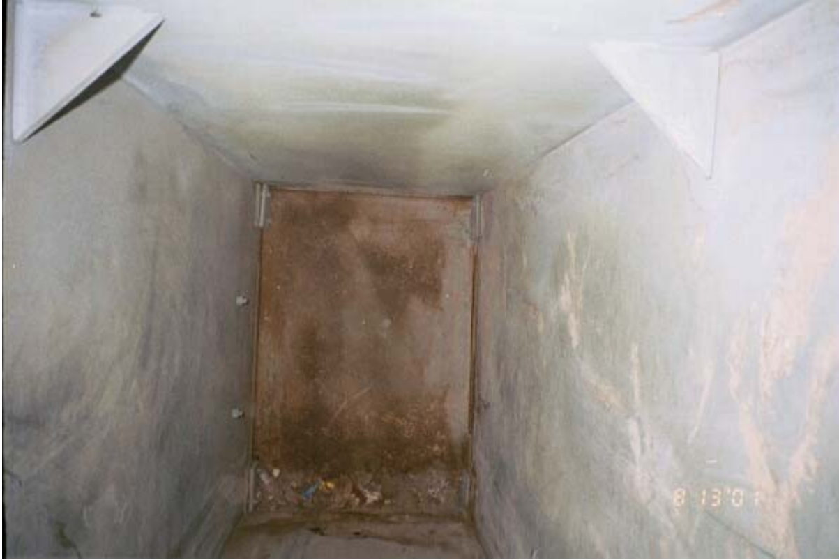
Arch rib interiors - typical surface rust at arch ends
