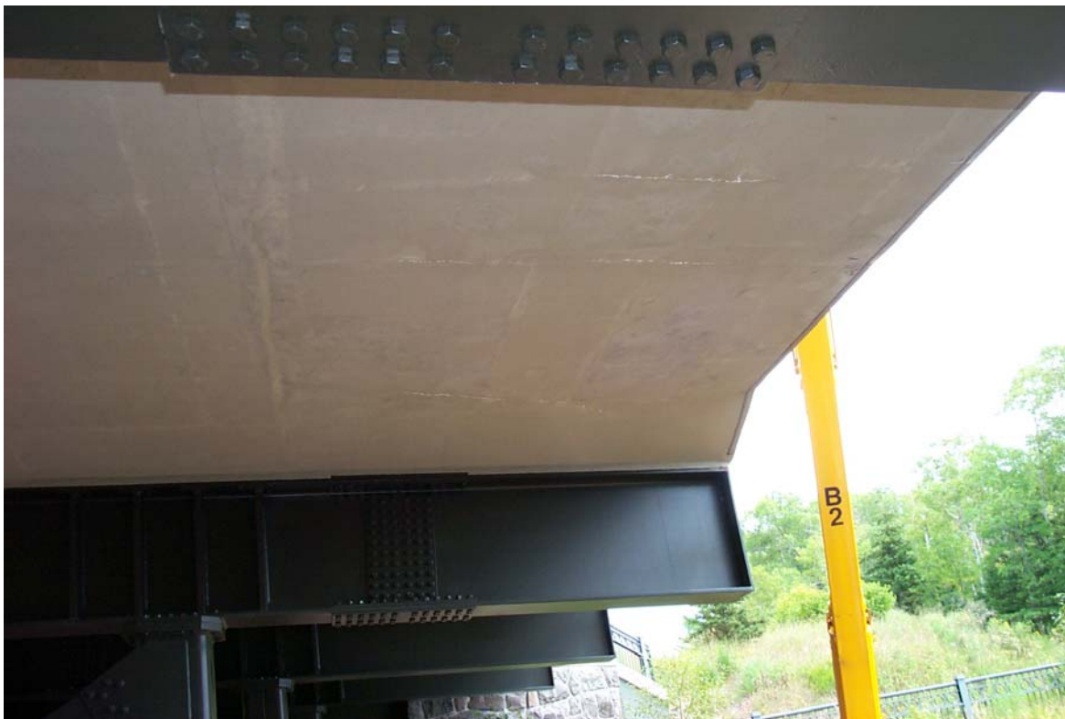
Photo #5: Light leaching cracks on underside of deck
