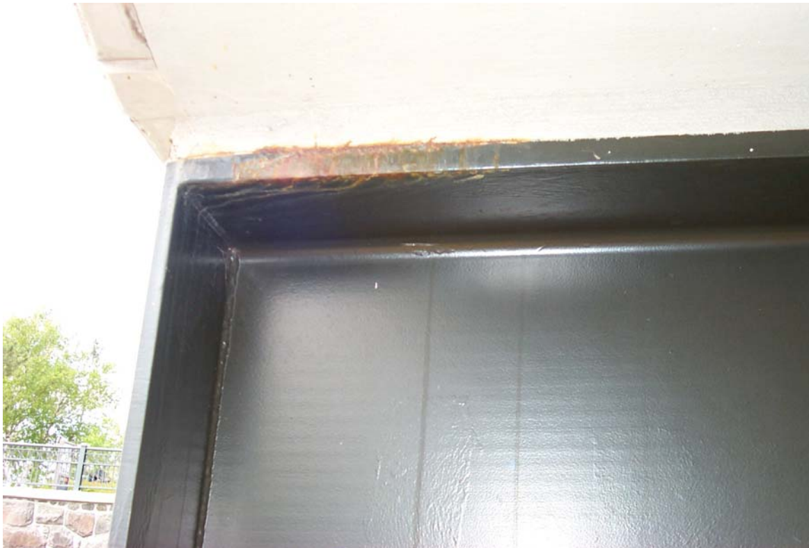
Photo #4: Minor corrosion on floorbeam end (typical)
