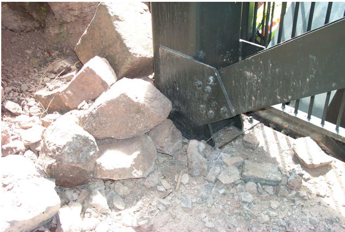
Photo #2: Debris at Pier #4 (east column)
