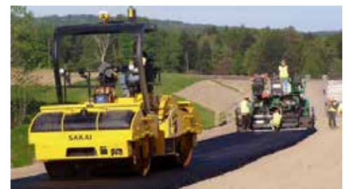
MnDOT is a leader in implementing intelligent compaction, a pavement roller technology that offers real-time quality monitoring.
