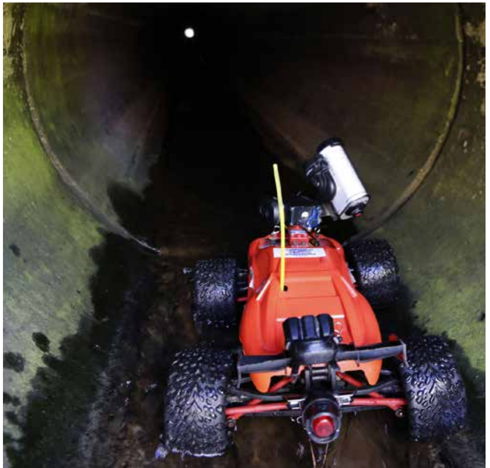
MnDOT District 6 developed the ingenious HIVE, which takes lights and a camera into the culvert and transmits data wirelessly to a tablet.
